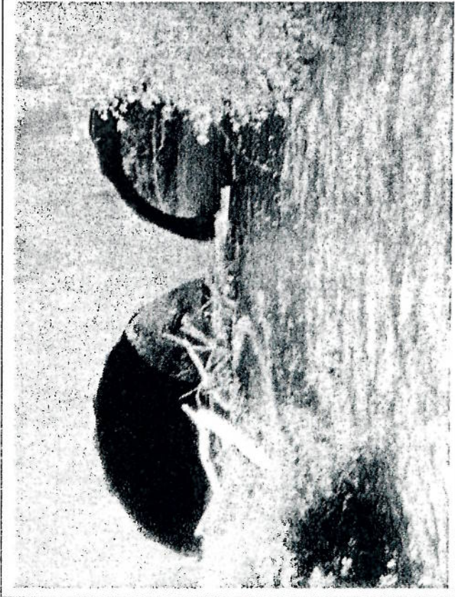
Photo # 3: EAST ELEVATION. NOTE DEBRIS AT INLET OF CELL 1.
