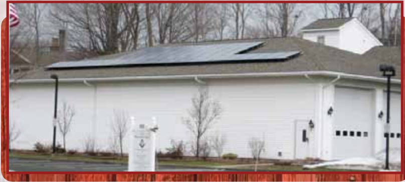
Nine kilowatt photovoltaic system on Fire Co. #2
