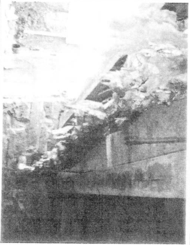
Photo # 6: 12 IN. WATER MAIN IN BAY 3 WITH WOODEN SUPPORT BRACKETS MISSING AND PIPE INSULATION DETACHED. THE ONLY SUPPORT FOR THE 30 FT. L. PIPE IS AT THE ABUTMENTS.
