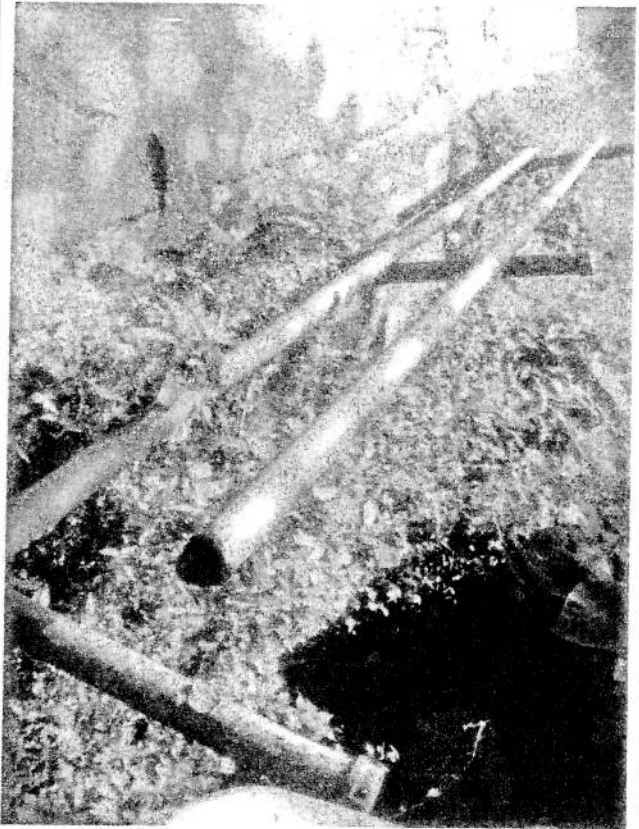
Photo # 5: LOOSE, RUSTED AND BROKEN PIPE RAIL AND POSTS AT THE SOUTH WEST APPROACH OFFERS NO PROTECTION.
