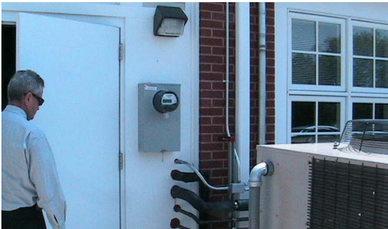
Fig 16: Side door to electrical room just below optimal roof location for solar panel.
