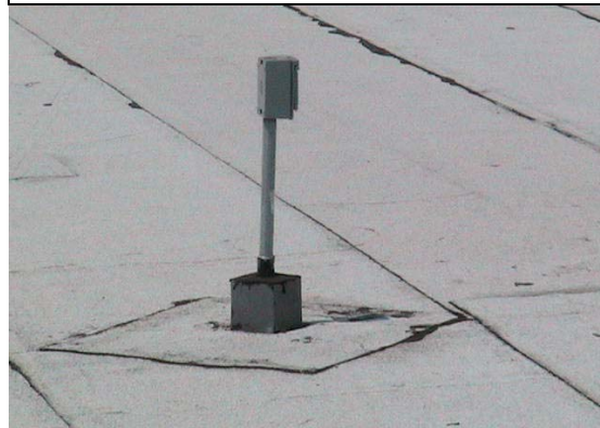
Fig 22: One of two AC outlets on "A" wing roof, close to array site.
