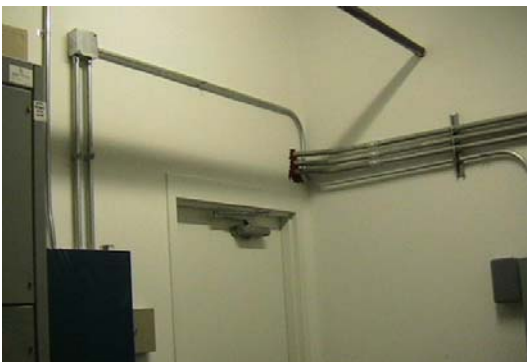
Figure 18: Conduit coming into electrical room
