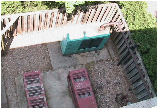
Fig 4: View of Generator from roof
