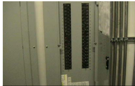
Figure 17: Circuit breaker box with spare breakers
