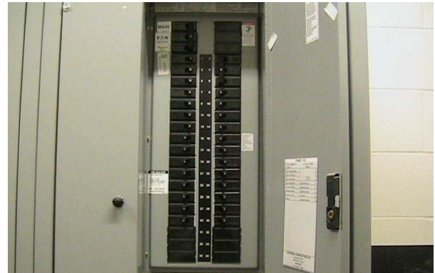
Fig 24: Several spare breakers available in CB boxes throughout the building.
