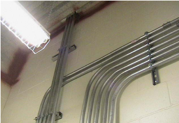
Fig 23: Conduit running from ceiling into second floor electrical closet.
