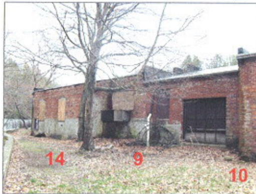
North side. Building 14 (Dye House, after 1922); Building 9 (Boiler House, ca. 1900); Building 10 (Engine Room, 1903).
