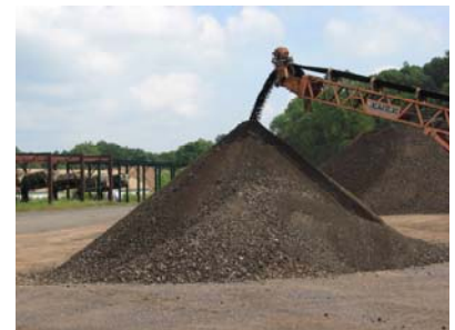
Raw aggregate waste materials lifted into crushing machine; resulting product reserved for future reuse
