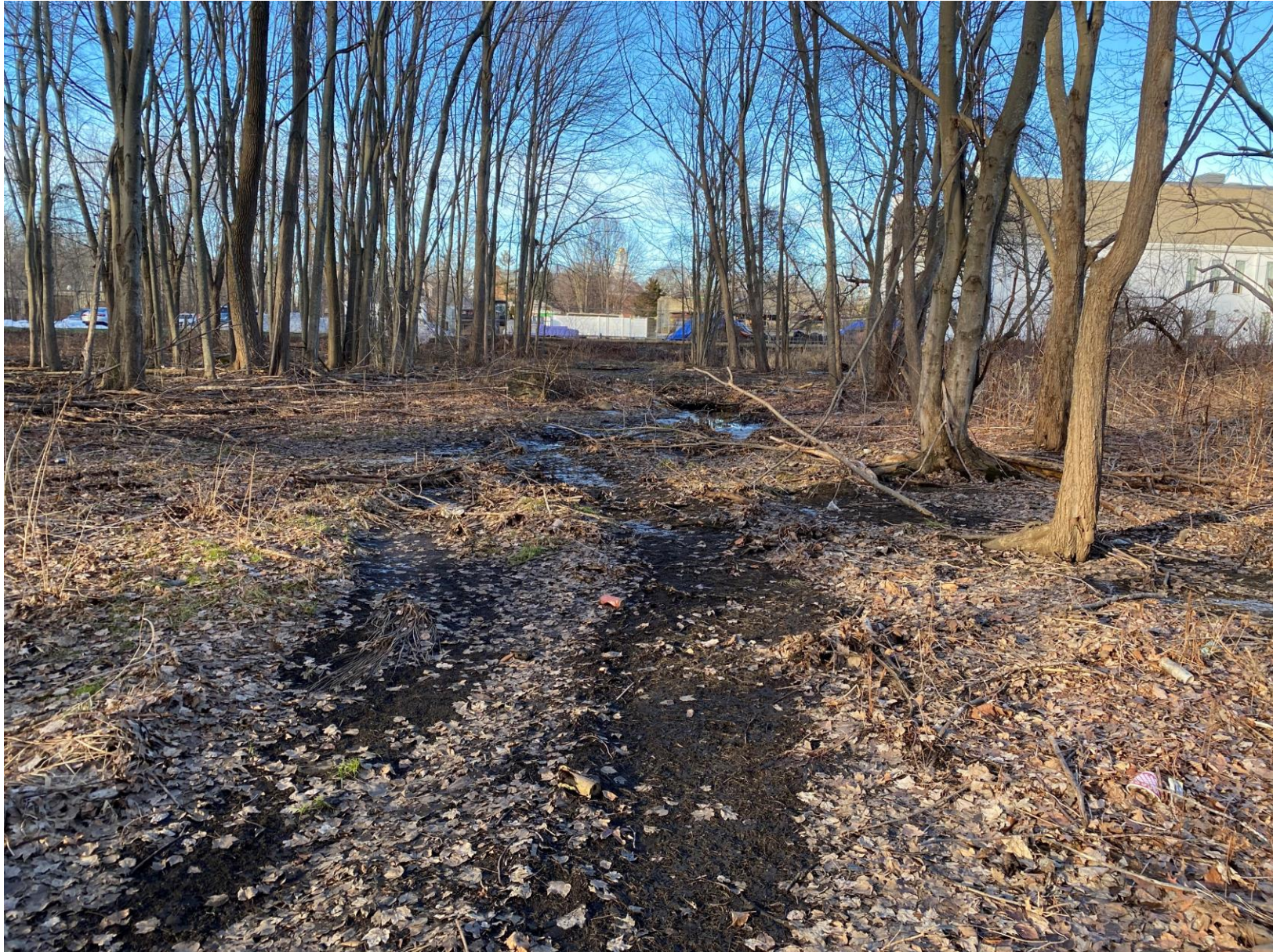
VIEW LOOKING NORTH ALONG SEWER EASEMENT SHOWING THE CLEARED EASEMENT AREA AND SURFACE FLOWS.
