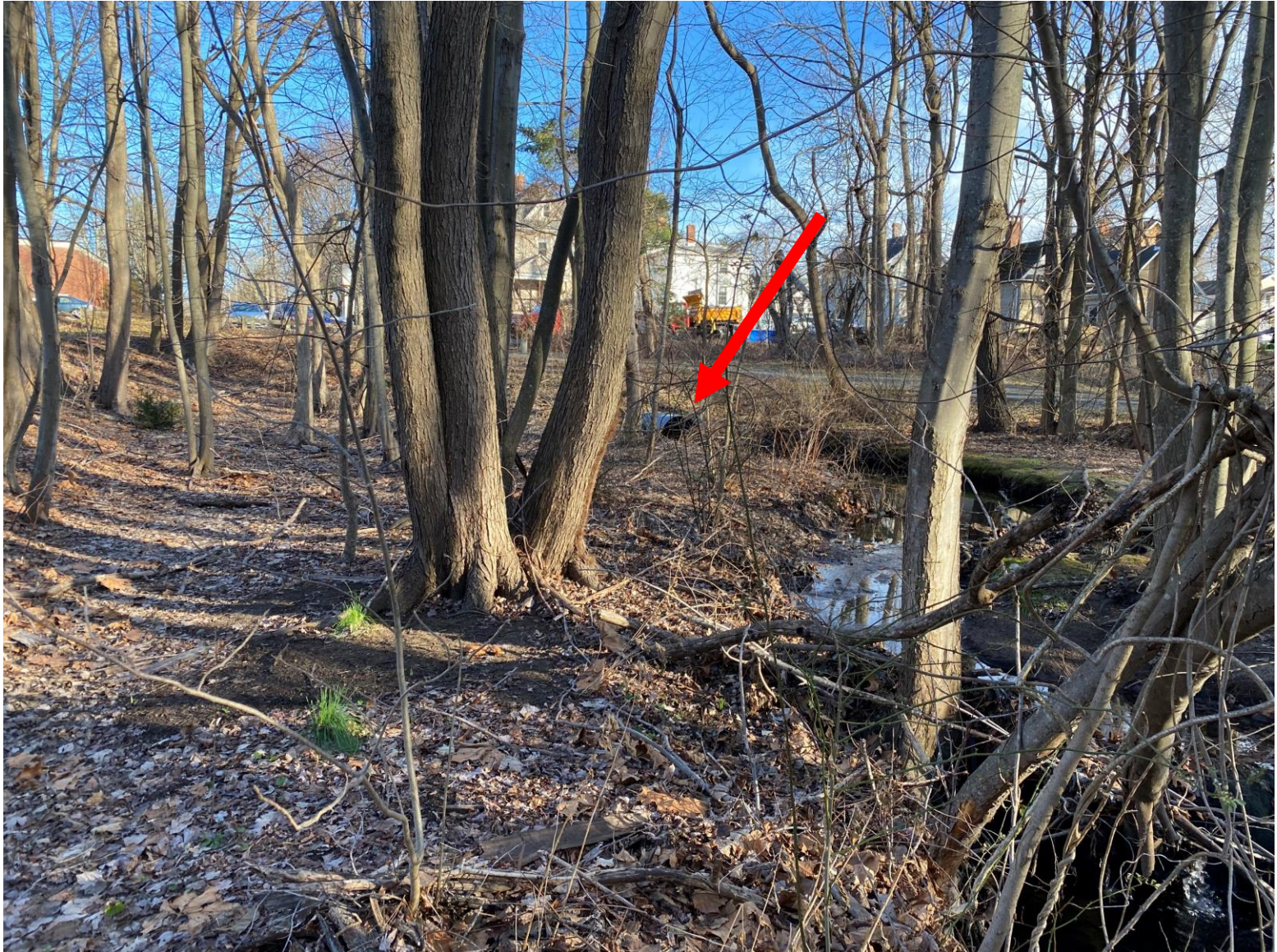
SOUTHERN PORTION OF SITE LOOKING EAST TOWARD CORRUGATED METAL PIPE OUTFALL (SEE ARROW) AND ASSOCIATED STREAMBED. NOTE FLOOD DEPOSITION IN FRONT OF MAPLE TREE CLUSTER IN LEFT CENTER OF PHOTOGRAPH.
