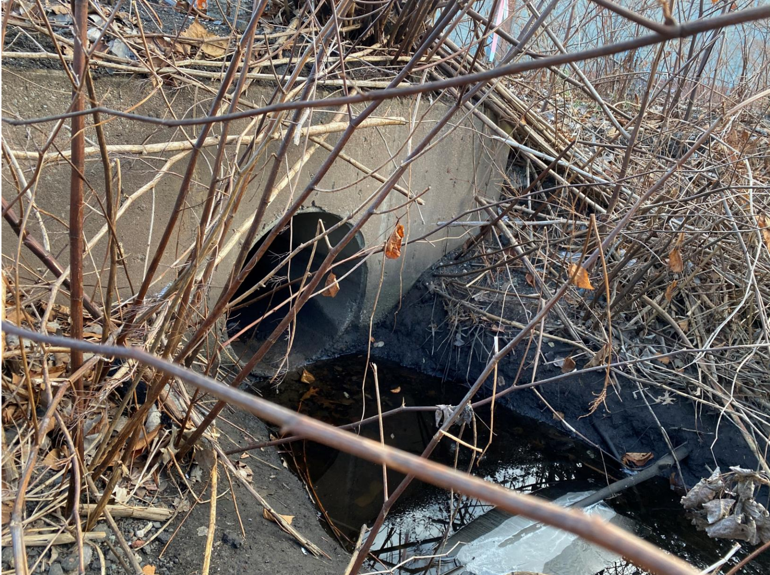
STORMWATER OUTFALL IN NORTHEASTERN PORTION OF WETLAND LOCATED WITHIN KNOTWEED STAND.
