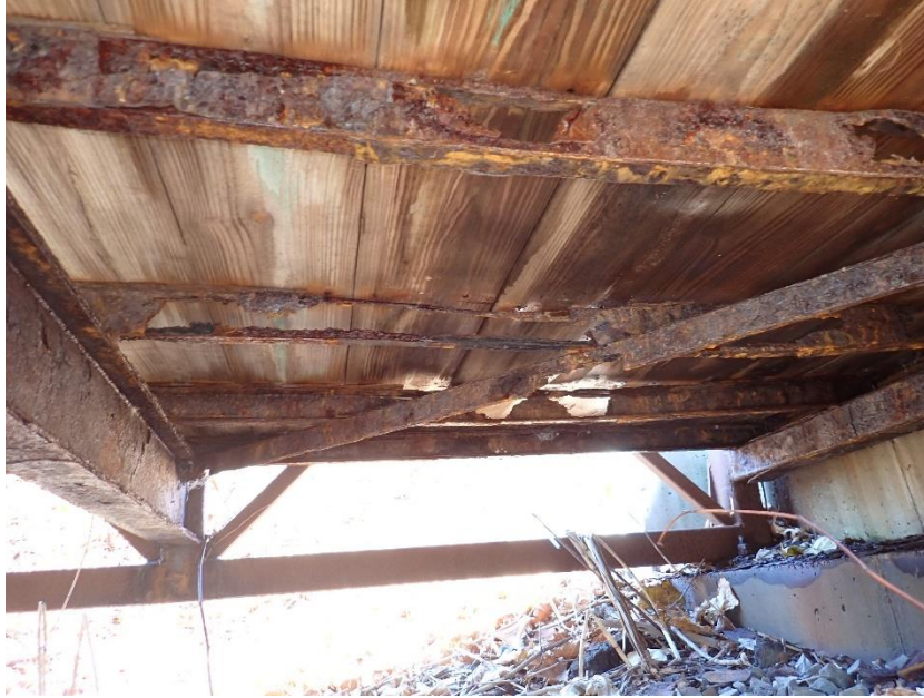
Steel stringers webs completely deteriorated at North abutment.
