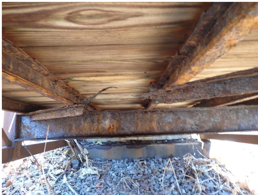
Fully deteriorated bracing angles
