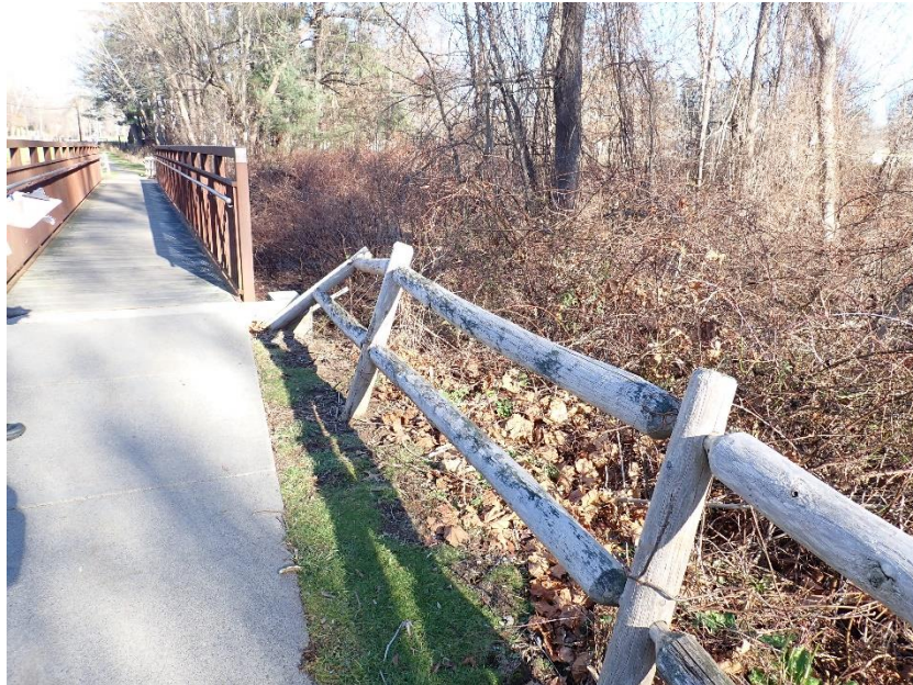
Northwest fence in failed condition
