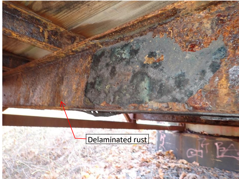
Typical section loss in the floor beam
