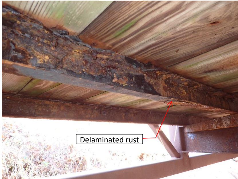
Typical section loss in the stringers
