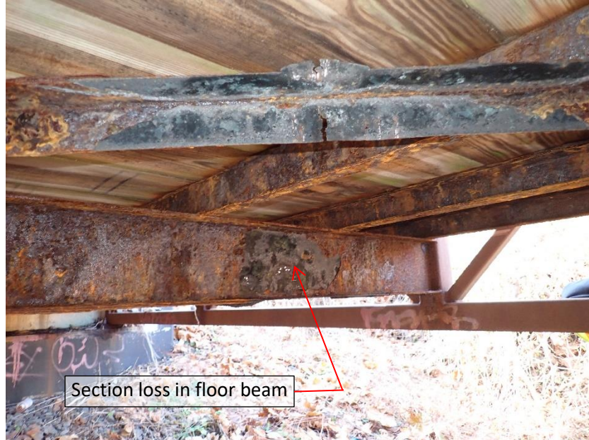
Packed rust, knife edging and section loss in framing
