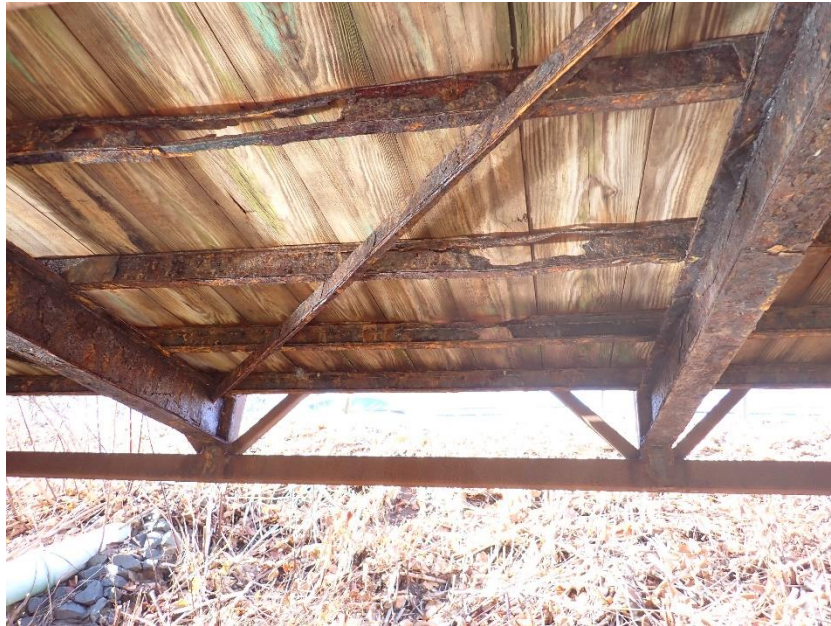
Steel stringers webs completely deteriorated.
