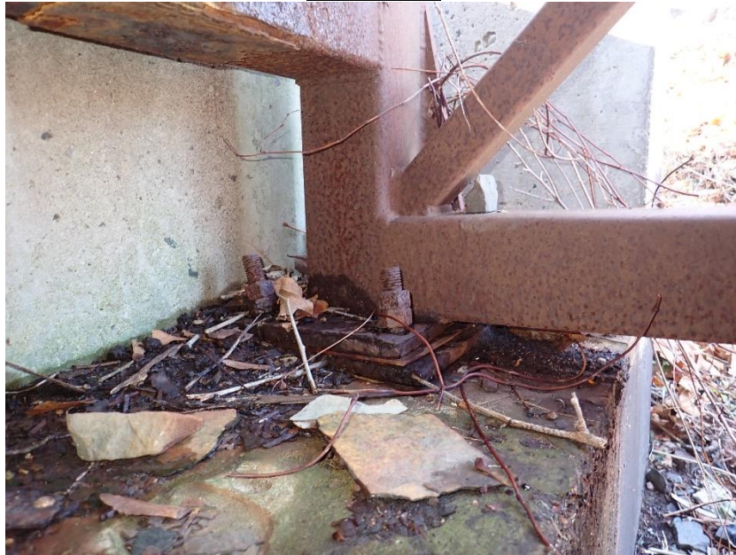
Typical Bearing, covered in dirt and debris.
