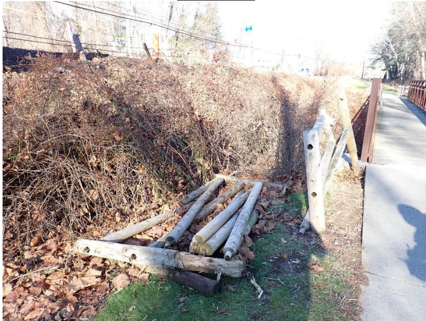
Southwest fence in failed condition
