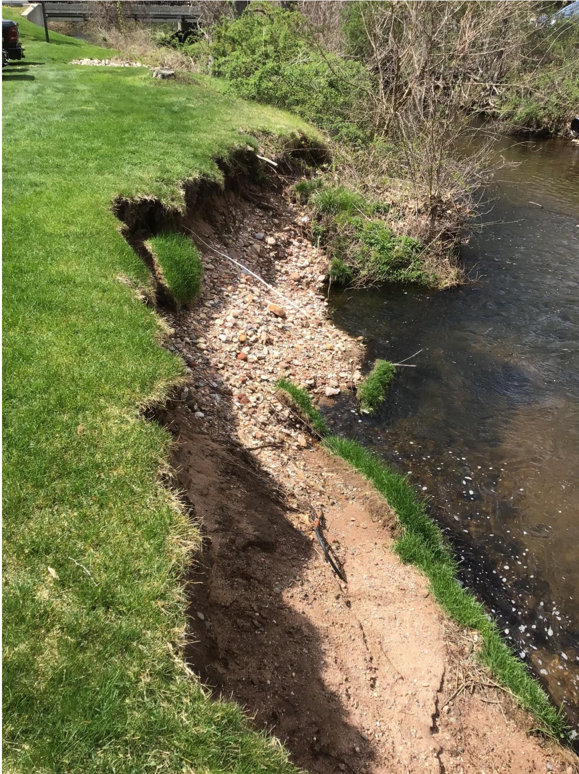
Photo 1: Looking west, lawn and stone eroding into the south bank of the brook. Irrigation tubing in the foreground.
