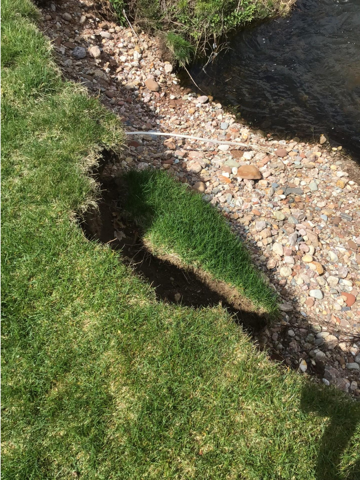
Photo 3: Undermining of established lawn, section breaking towards the brook
