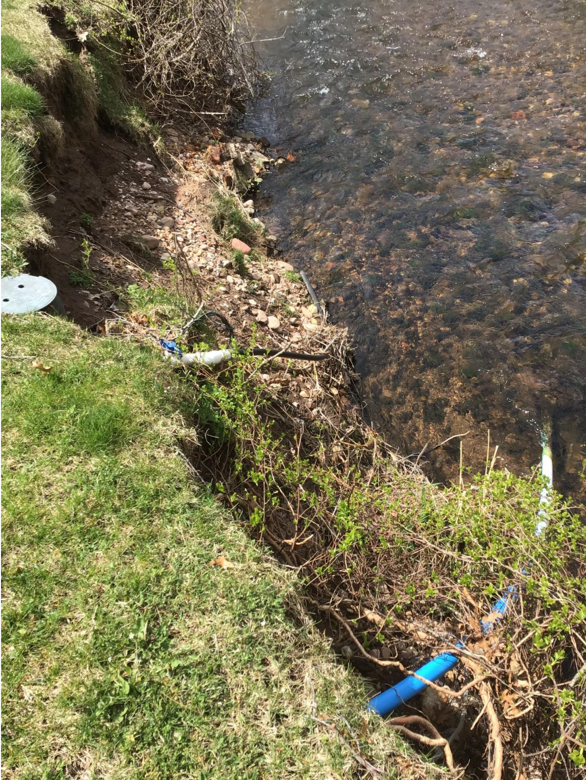
Photo 2: Irrigation tubing, valve and control box.
