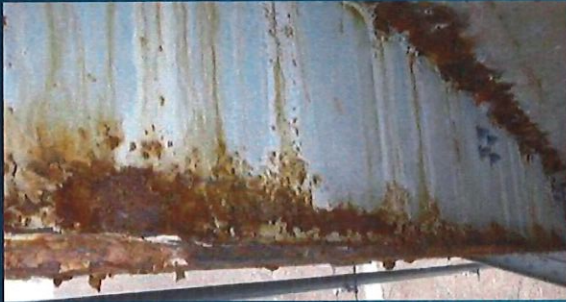
Corrosion and section loss on first interior stringers
