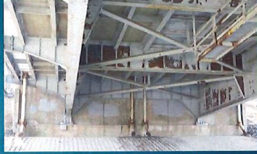
Typical paint system failure and girder corrosion
