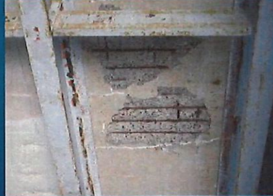
Spall on underside of deck
