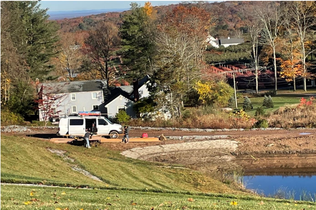
Photo taken by S. Simone, October 31, 2023: Workers at 150 Chatham Hill Rd possibly constructing wood forms for concrete.
