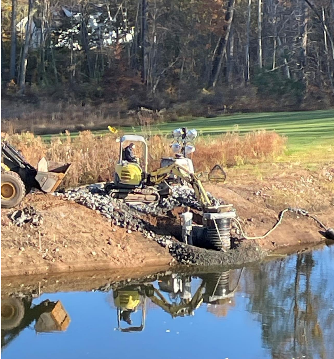
Photo taken by S. Simone, October 31, 2023: Excavation at pond, 150 Chatham Hill Rd. Dewatering pump in lower right. Utility lighting (unknown if used to power the pump, or work planned into the night).
