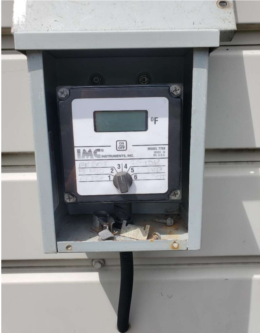
Existing Temperature Monitoring Controller – Upgrade for use on all (3) Burn Rooms
