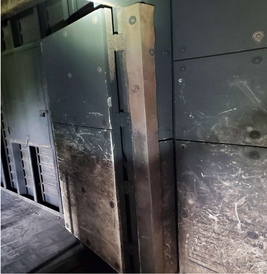
Metal Door Edge Protection, replacement on all burn room doors, full height of door.
