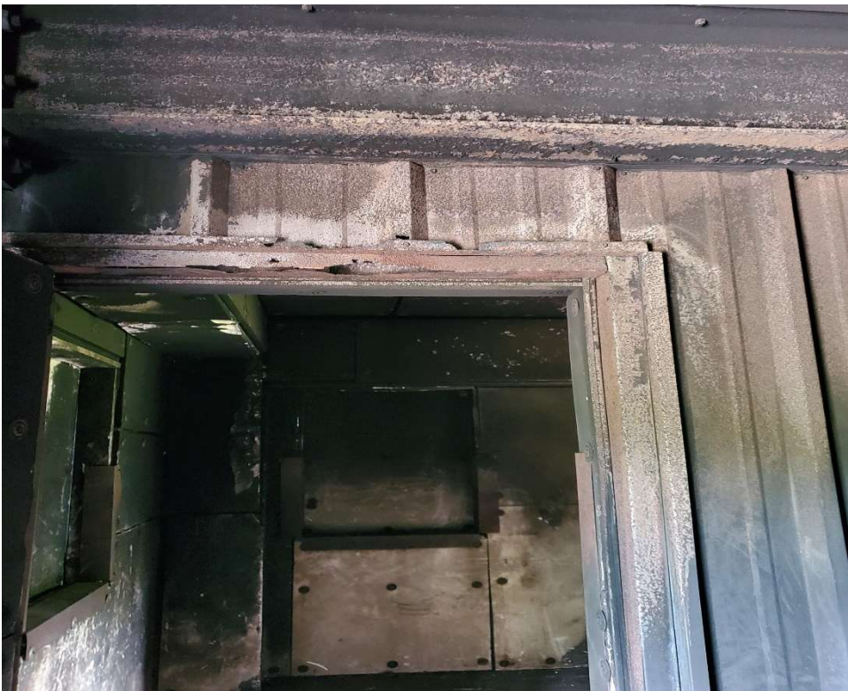
Existing Second Floor “A” side Burn Room Door – Frame and Wall Replacement
