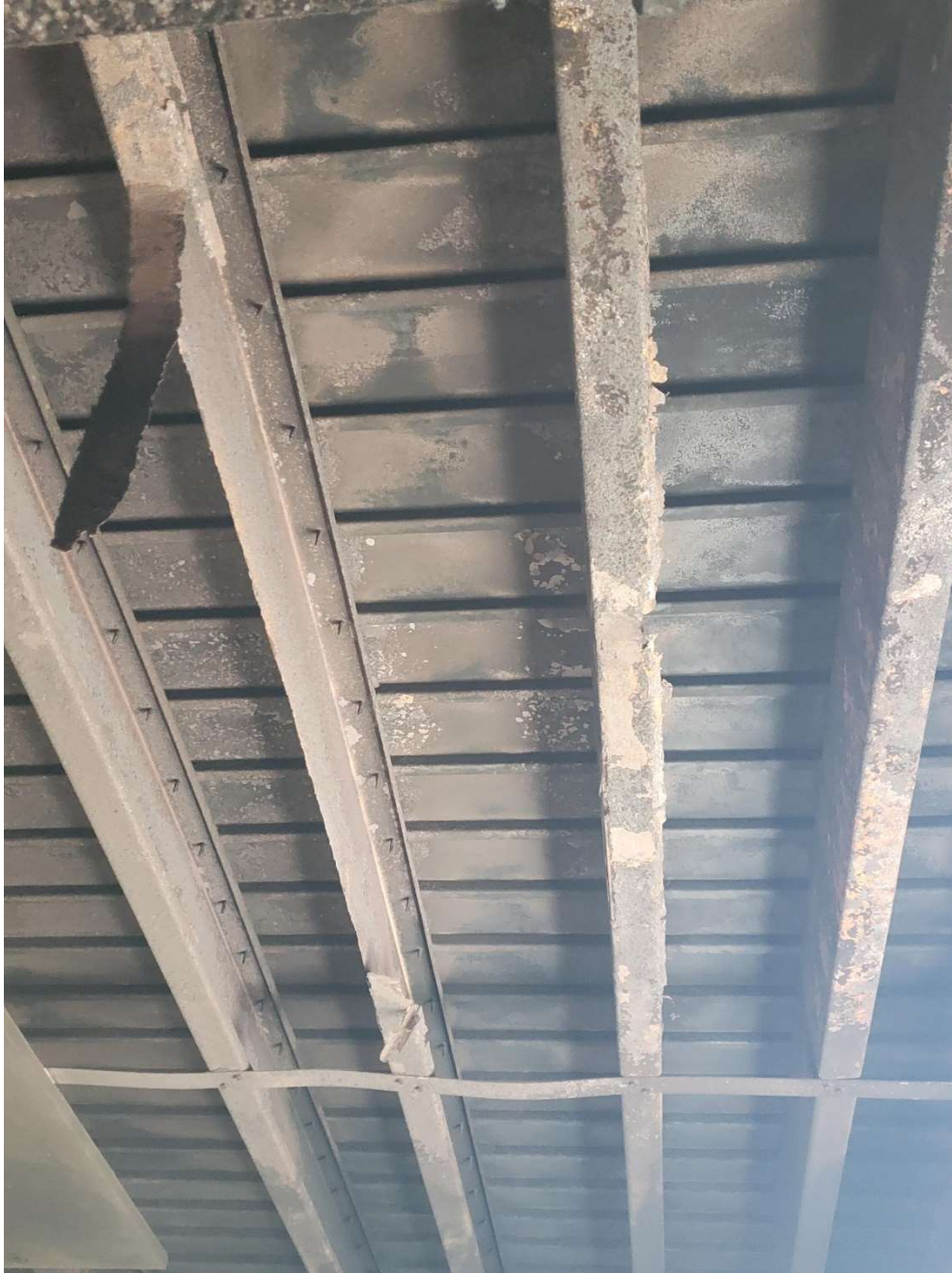
Three (3) floor joists for the second-floor need replacement. Joists are located outside the first floor burn room.
