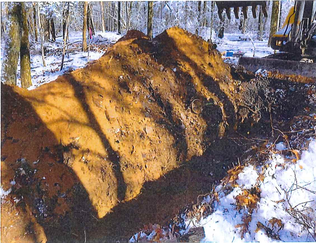
Figure 3: Solid waste found in TP-L9, south of TP-L1. Both test pits are adjacent to the access path.
