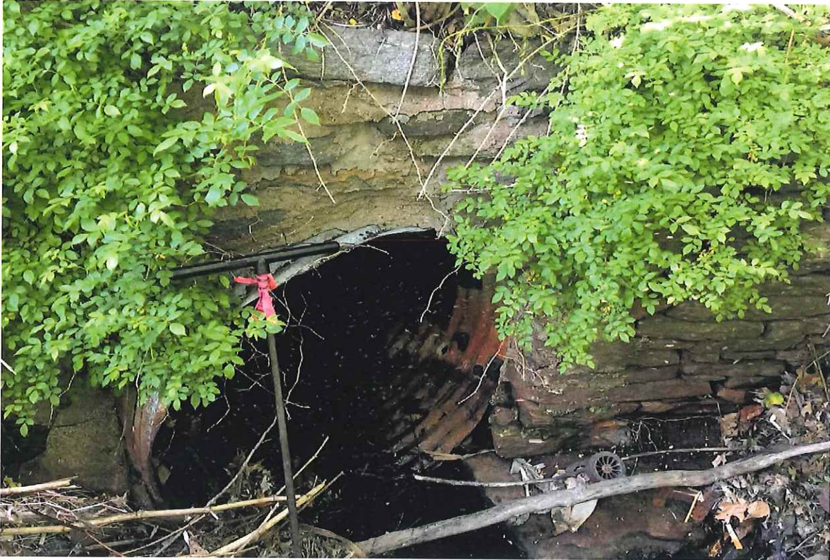
Photo 3: View of existing culvert on 2800 Main Street parcel conveying flows south under Spring Street looking west.
