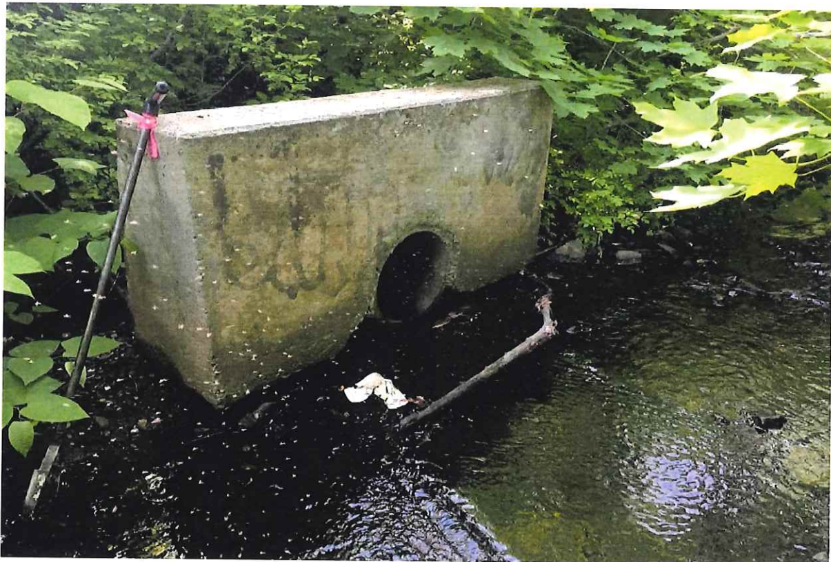
Photo 6: View of direct stormwater discharge into watercourse from Dairy Queen property looking northwest.
