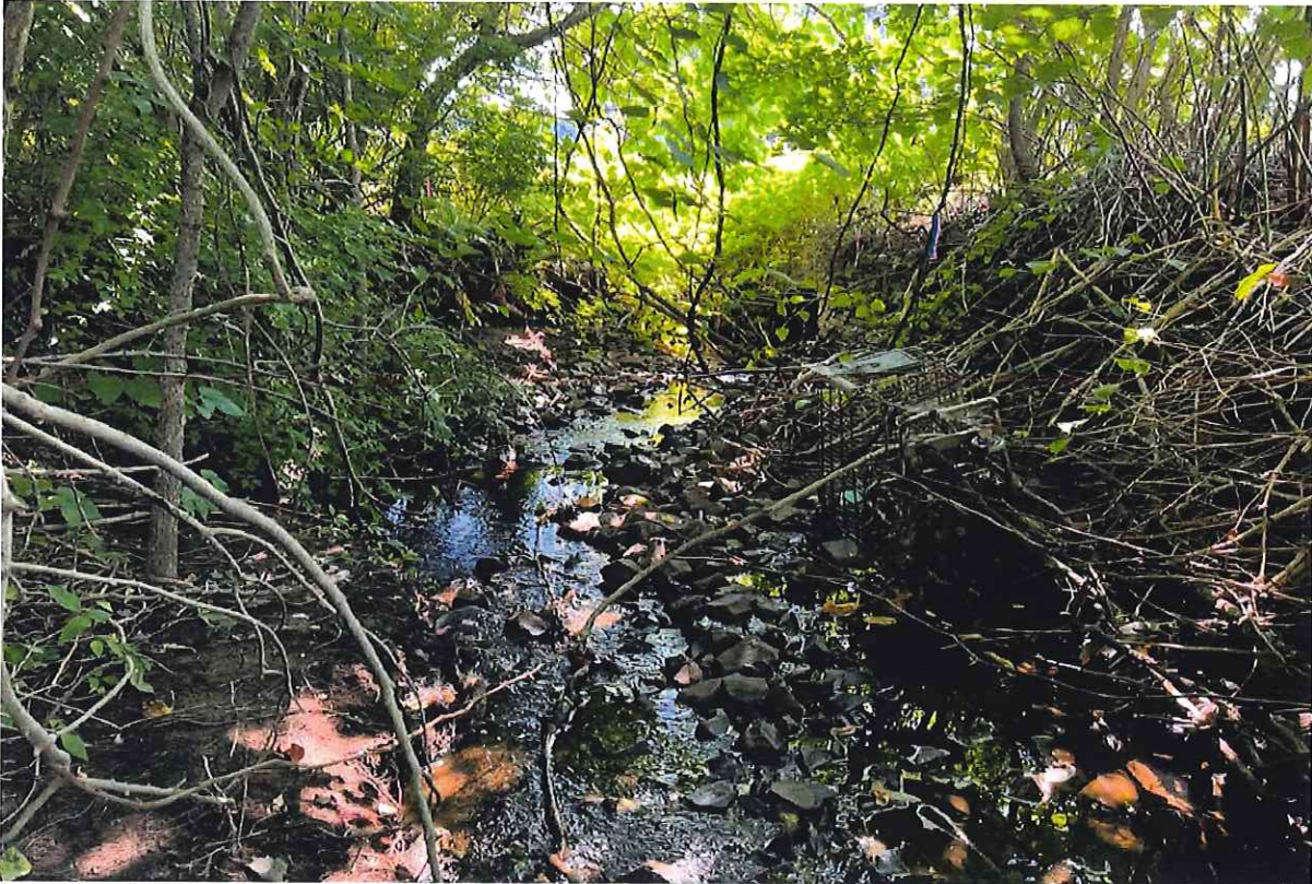
Photo 1: View of Wetland 1 watercourse channel with stone armoring looking south at 48-inch CMP culvert on 2800 Main Street in background.
