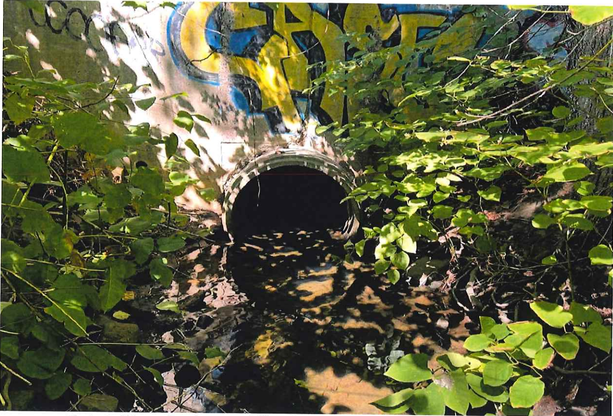
Photo 5: View of culvert outfall and headwall of watercourse at south end of Griswold Shoppes property, looking north.
