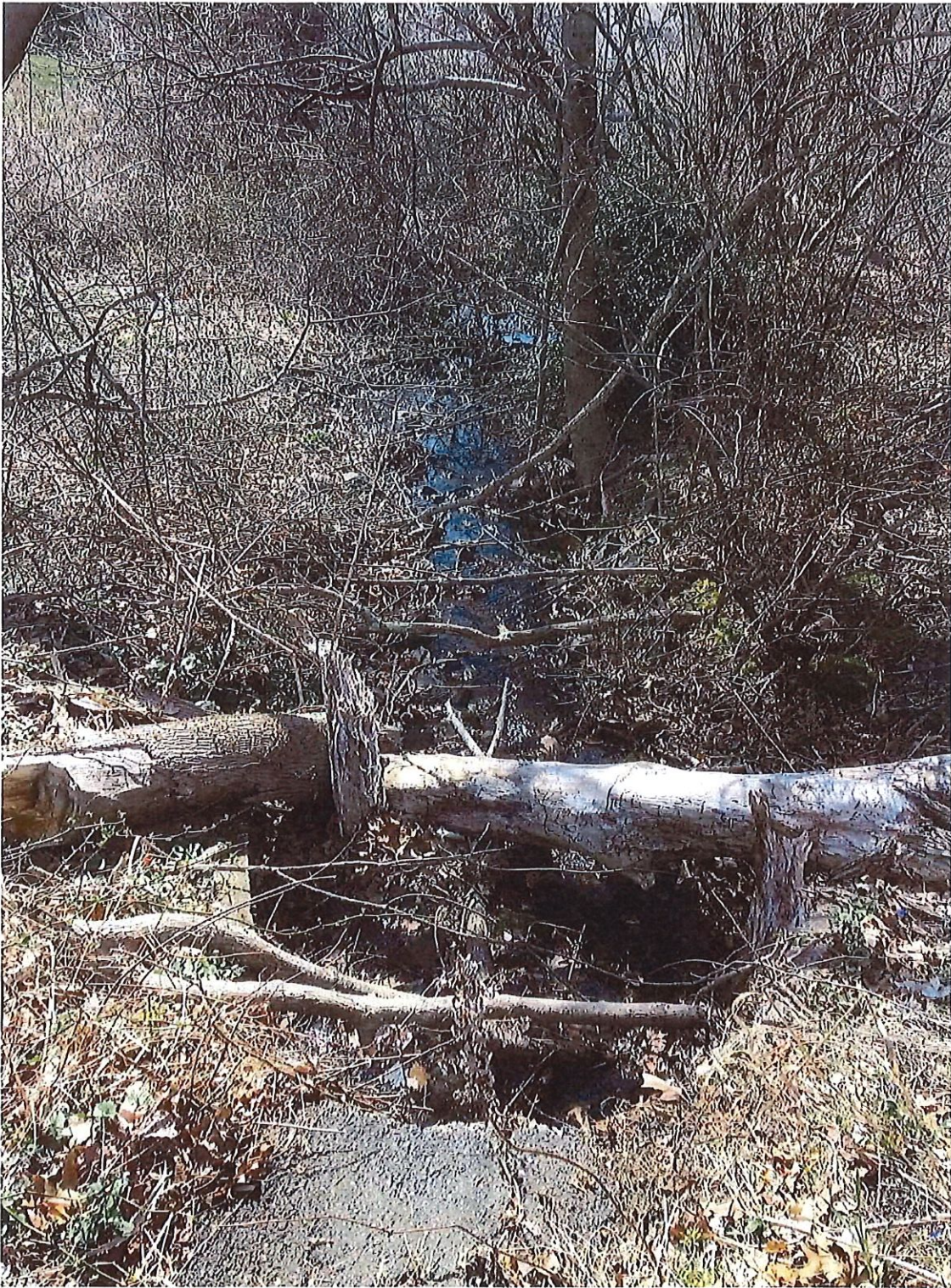
Photo 4, April 4, 2023: Watercourse flowing from under Ledgewood Dr into conservation easement.
