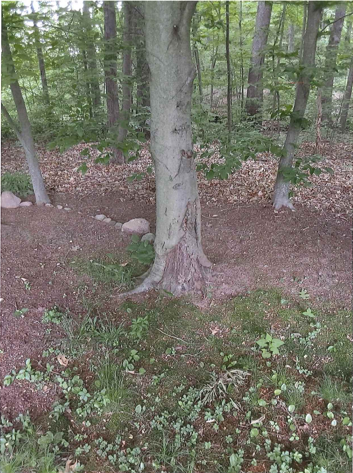
Photograph 6: Tree #4 showing mechanical damage to the root flare. This tree has a high likelihood of failure due to the defect and assigned a Moderate risk rating due to the distance from a target. Mitigation would include Monitoring and health care treatment. If Moderate risk is acceptable, retain and treat or perform removal to eliminate the risk.
