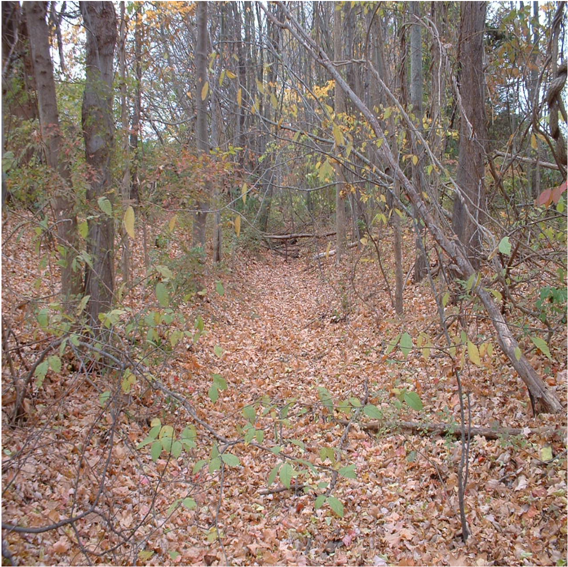
Looking east in the existing storm water swale. Photograph taken on 10-29-13. No signs of erosion.
