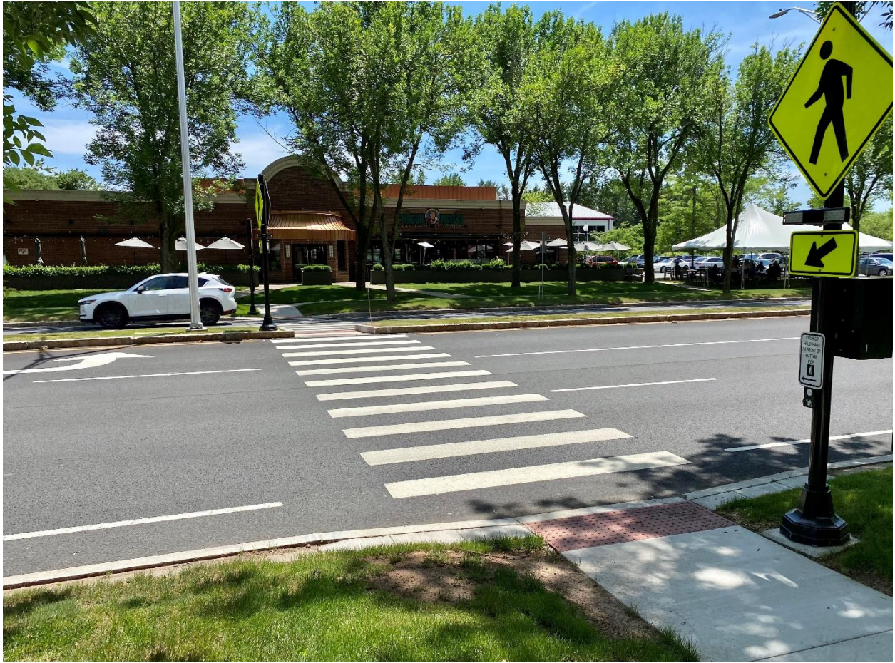
One of three newly installed RRFB signalized pedestrian crossings. Pedestrian phases also added to three existing signalized intersections.
