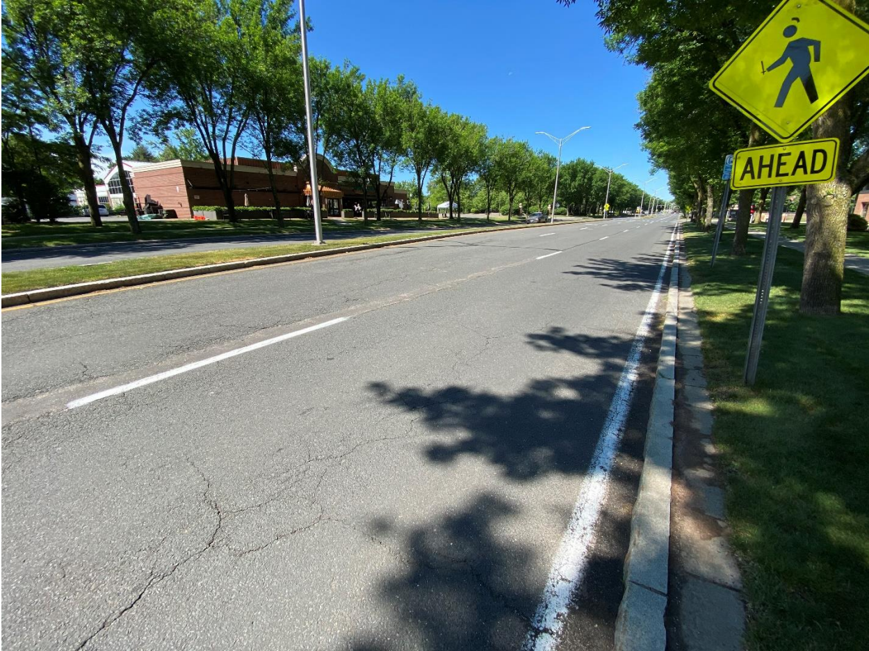
Absence of shoulder width prior to construction
