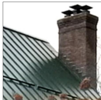
Standing seam material with snow guards
