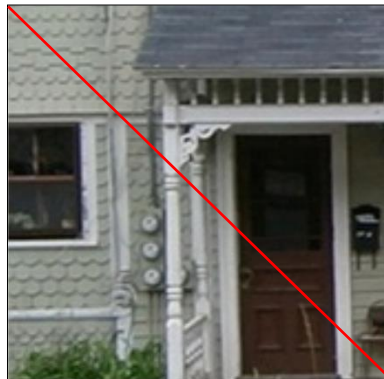
No electrical equipment on front facade
