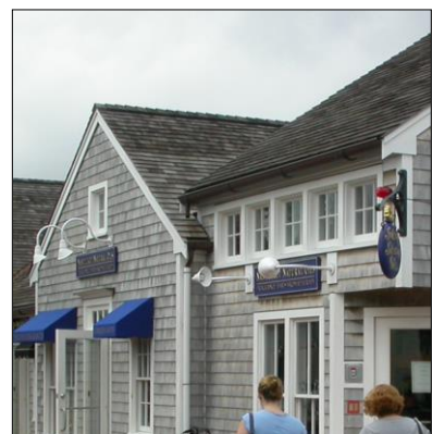
Wall sign lighting
