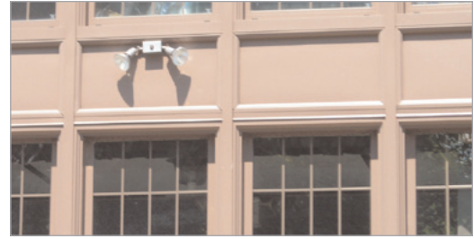
Floodlights result in unwanted glare and energy inefficiencies.
