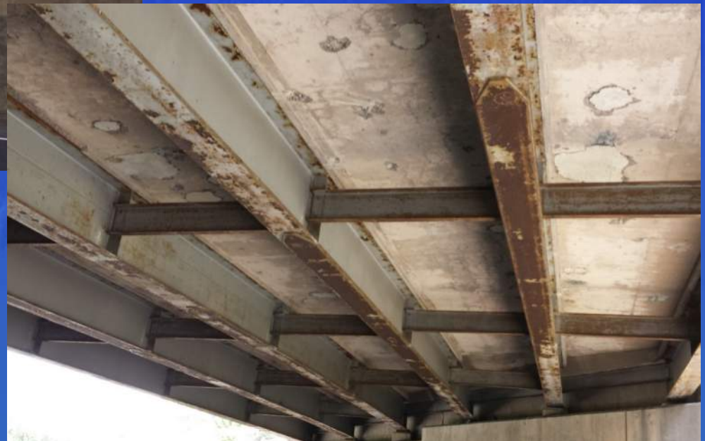
Typical Deterioration Seen on Underside of Deck
