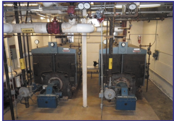
Boilers to be replaced at Town Hall.
