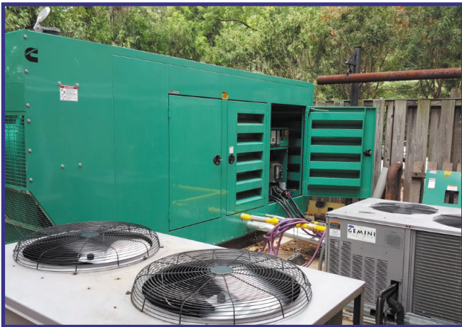
New generator at Town Hall.
