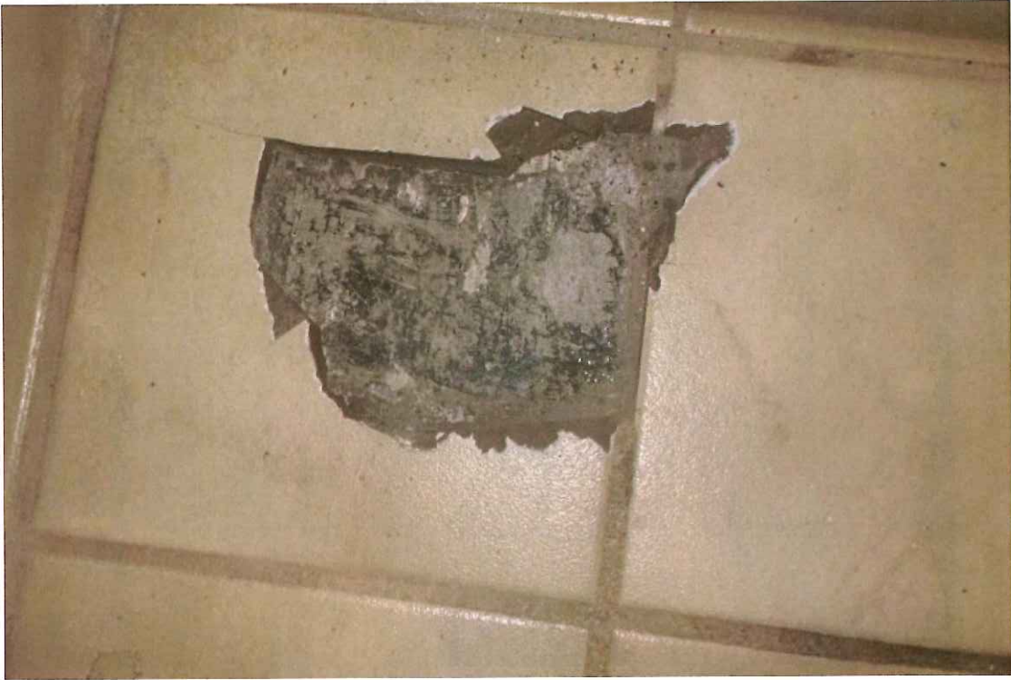
Black mastic under ceramic floor tile system bathroom #2 shop area
