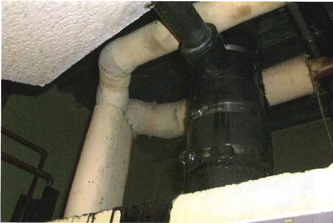
Muddied pipe insulation above drop ceiling bathroom #2 shop area
