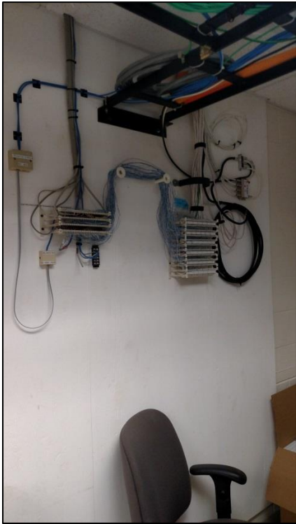
2143 Main Street (Server Room)
