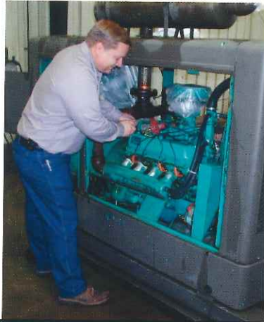
Robert Planeta, Town Electrician, working on the new air conditioning system in the Academy School cafeteria.
