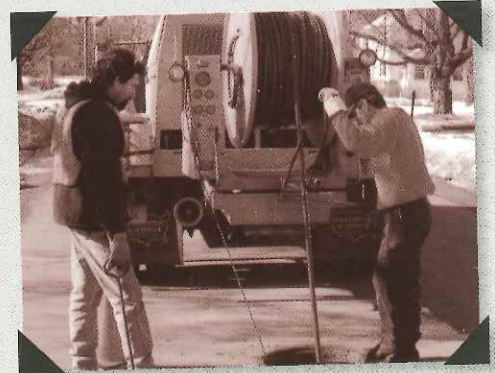
Highway Division workers Brett Somers and Ron Morrone flush and clean a sewer manhole and line.
