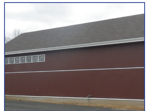
Pictured from top to bottom, the progressive construction of the new Facilities Barn between June and November of 2015.
