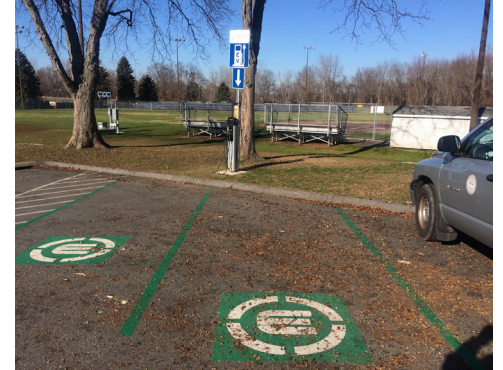
Electric Vehicle Charging Station installed in Town Hall complex.
