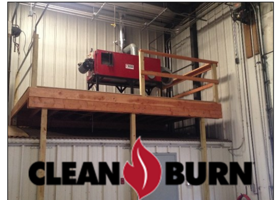
Waste Oil Heater at the Vehicle Maintenance Facility. The Unit is stored on an elevated platform and connected and fed by oil tanks stored below.
