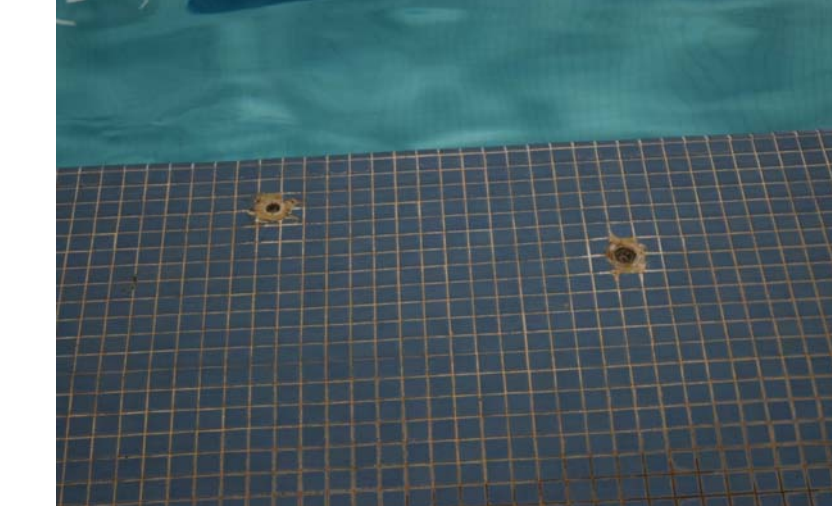
13.7 Remove broken tile along length of crack, repair cracked mortar bed, remove loose material;
