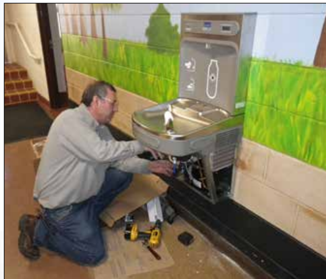
Senior Building Maintainer Jon Gilroy installs a water bottle filler at Academy Building, one of many throughout Town facilities that have kept more than 50,000 plastic bottles out of the waste stream.
