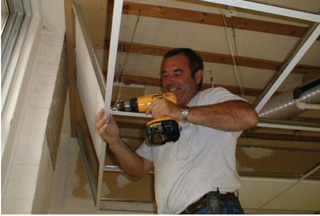
John Gilroy, Senior Building Maintainer, installs a new suspended ceiling in Town Hall.
